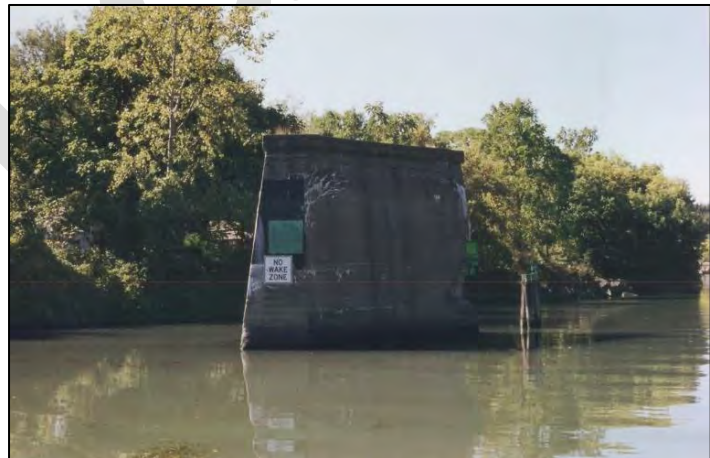
Some potential hazards can be a concern to boaters along the Canal like this abutment west of Bear Ridge Road.
