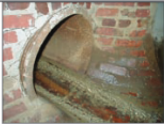
Bacterial growth at this outfall indicates nutrient enrichment and a likely sewage source.
