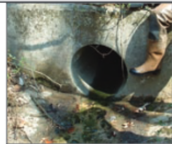
The drainage to this outfall most likely has a high nutrient concentration. The cause may be an illicit discharge, but may be excessive use of lawn chemicals.
