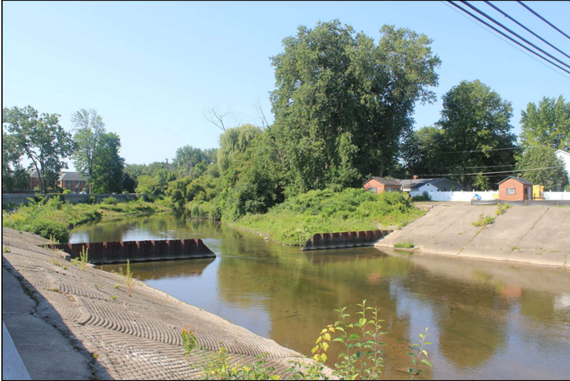
Source: Town of Amherst USACE flood control project. Town Staff Photo Taken August 24, 2018.
