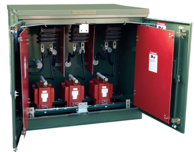
Metering Transformer Compartment With Barriers Secured Open
