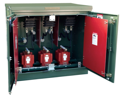
Metering Transformer Compartment With Barriers Secured Open
