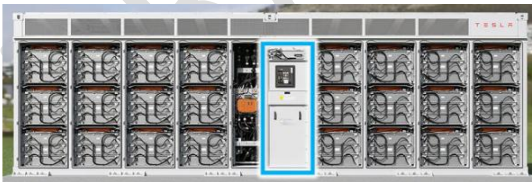
Figure 6: MP2XL Cabinet Interior
