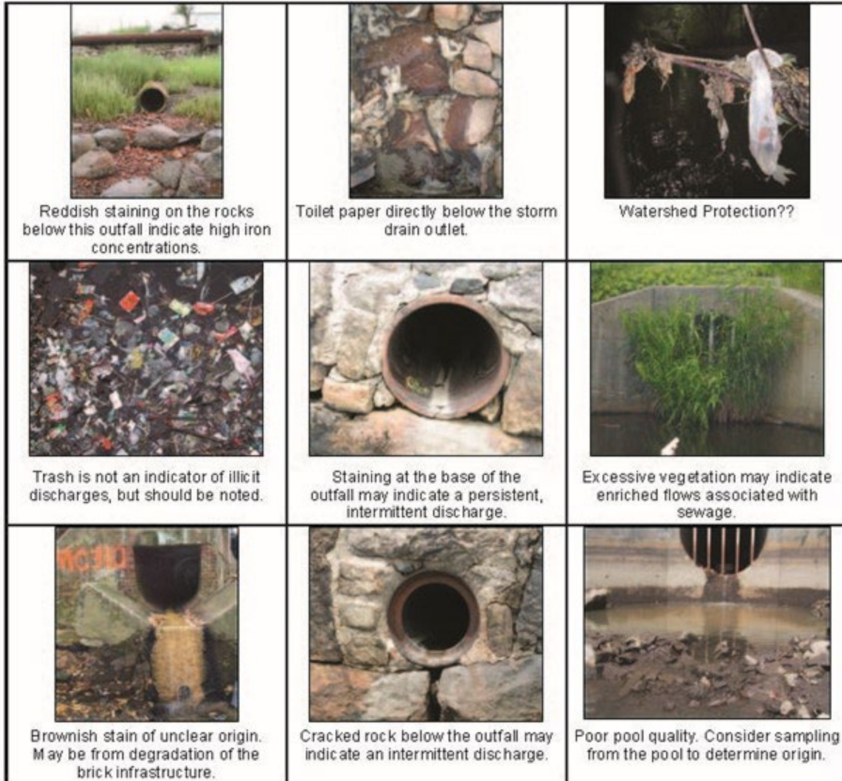
Figure 39: Typical Findings at Both Flowing and Non-Flowing Outfalls
